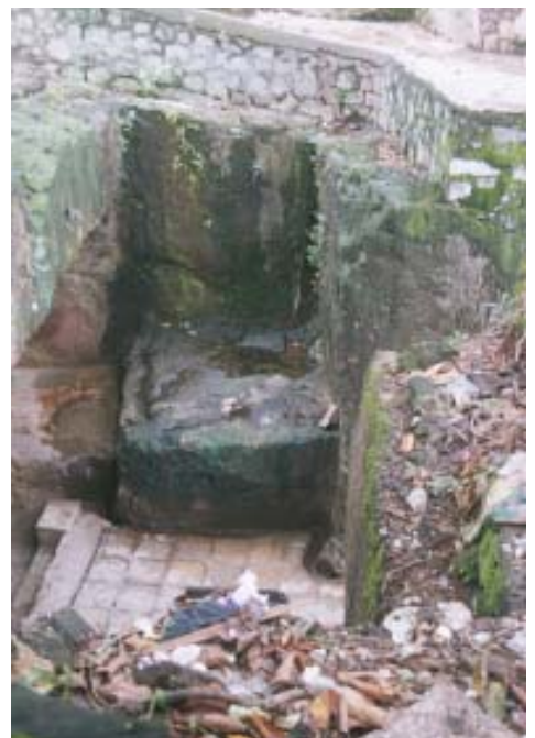
DETAIL SHOWING THE RUINED CONDITION
